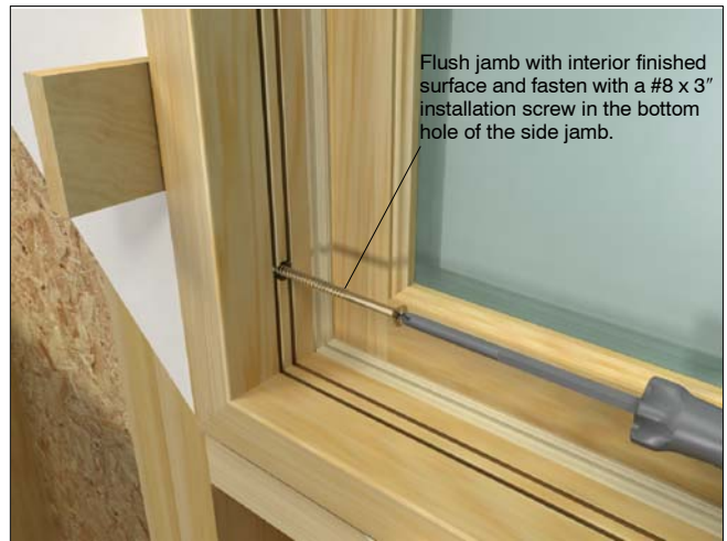
Figure 6: Flush with interior surface and screw through lower end of side jamb
